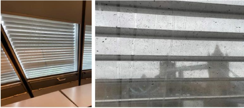
These images show the existing louvre system and the view through to Tower Bridge .
